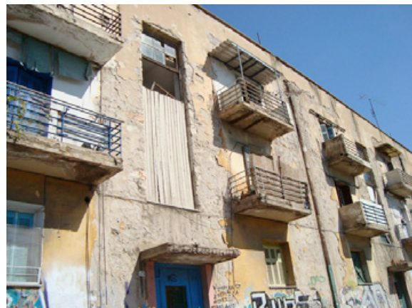
Aspect of one of the buildings of the former refugee housing complex. Deterioration and neglect are apparent. Source: personal archive.
